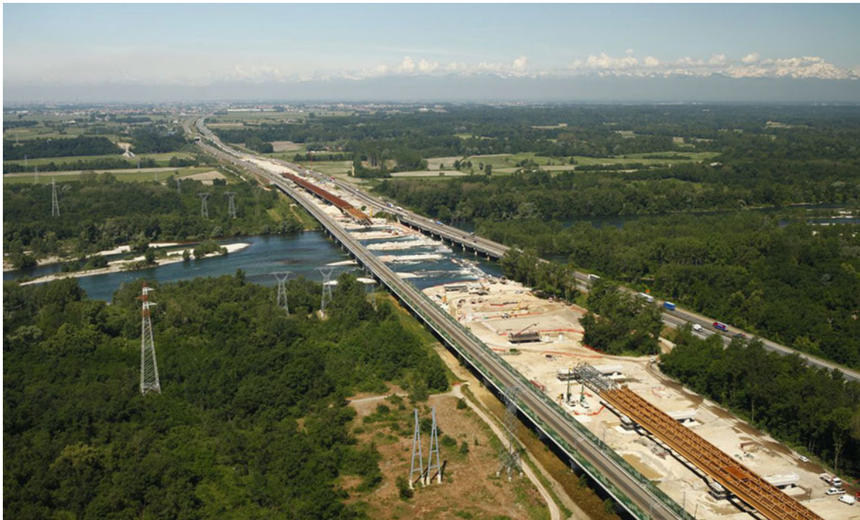
Figure 2 | The creation of new infrastructures improves connectivity between northeastern Piedmont and the Milan metropolitan area. The picture shows the road expansion work on the Milan-Turin motorway and the high-speed/capacity railway along the Ticino River, which draws the boundary between Piedmont and Lombardy.
