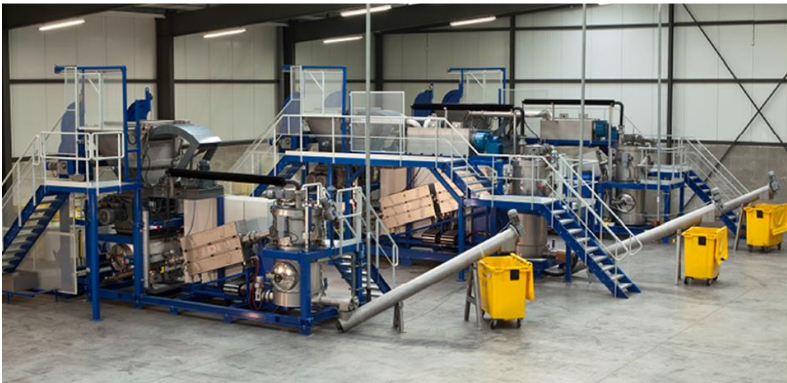
Figure 18 Installation machines Ecosteryl (Source : https://cosmolys.com/solution-globale/ )
